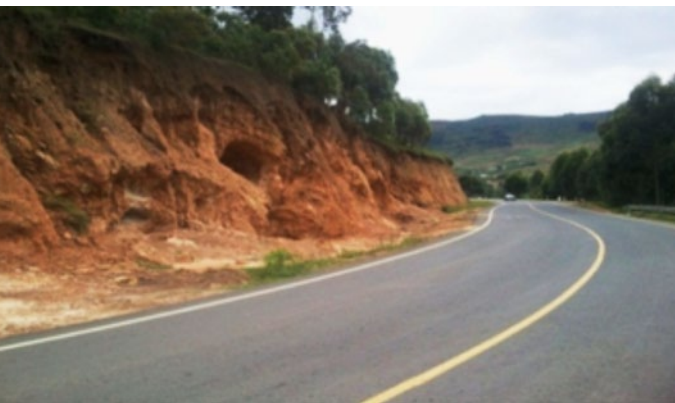
Photo 1 - Erosion on the Kabale-Kisoro road in South-western Uganda
